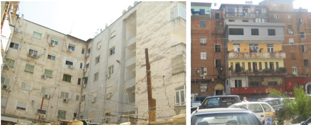
Figure 1. Building constructed after '90. Facade degradation.
