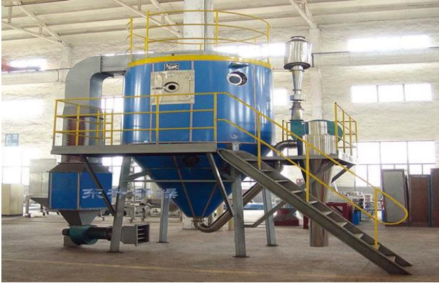
Fig. 3. Industrial spray dryer
