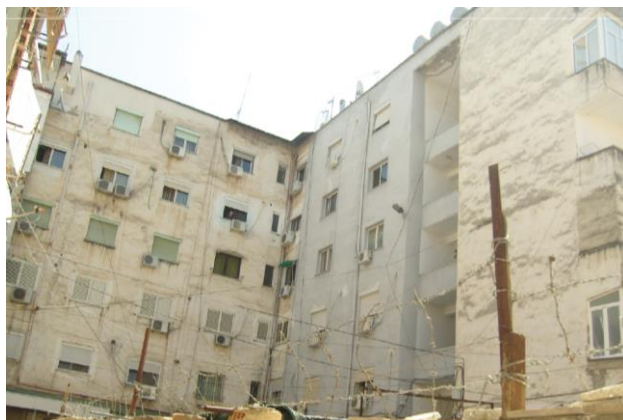
Figure 1. Building constructed after '90. Facade degradation. trasformation
